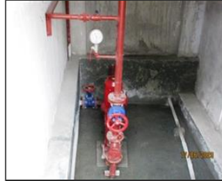
Photo of fire safety equipment Fire Pump.JPG
