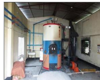
External photo(s) of the production unit(s) Waste Incineration Boiler.JPG
