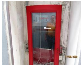
Photo of fire safety equipment Fire Control Panel.JPG
