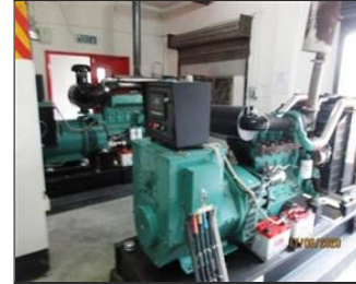
External photo(s) of the production unit(s) Generator.JPG
