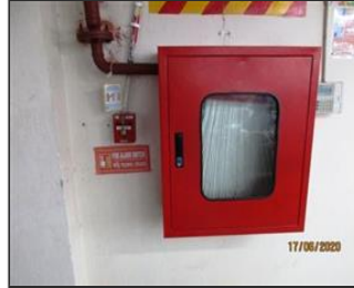
Photo of fire safety equipment Fire hose pipe box.JPG
