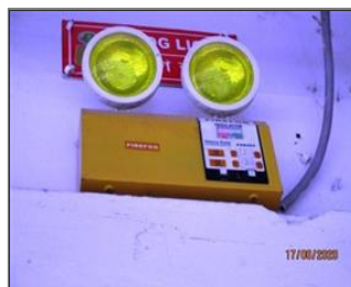
Photo of fire safety equipment Industrial battery backup fog light.JPG
