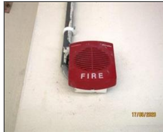
Photo of fire safety equipment Fire Alarm.JPG
