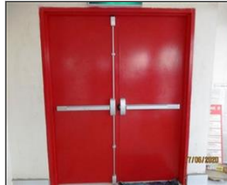
Photo of fire safety equipment Fire Resistance Door.JPG
