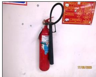
Photo of fire safety equipment Fire Extinguisher.JPG
