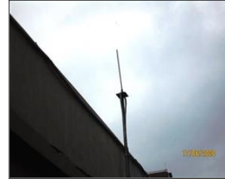
External photo(s) of the production unit(s) Lighting protection system.JPG
